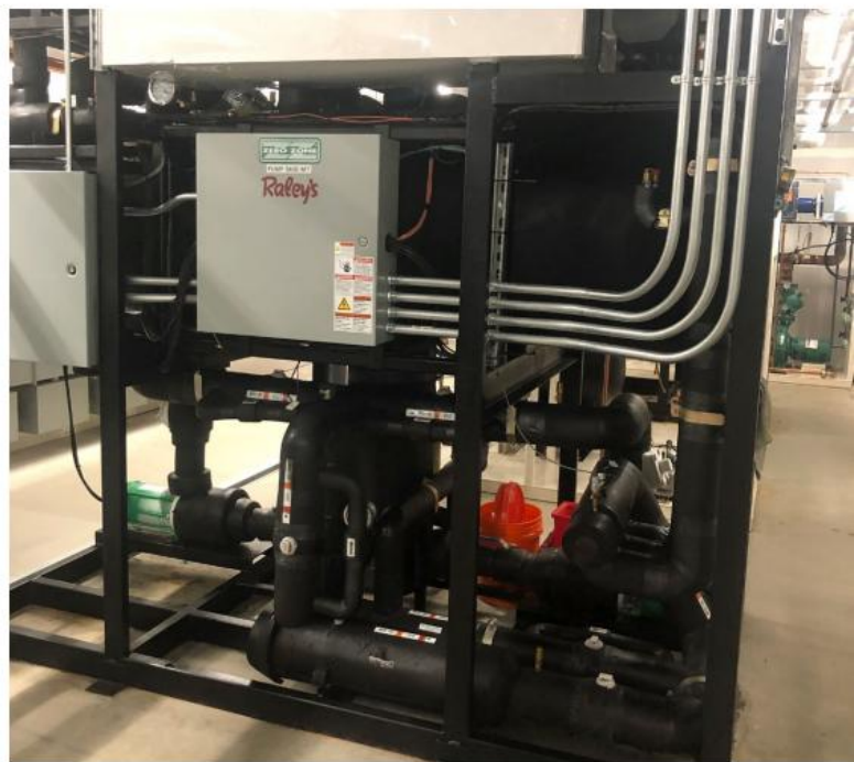
CO 2 overfeed rack
