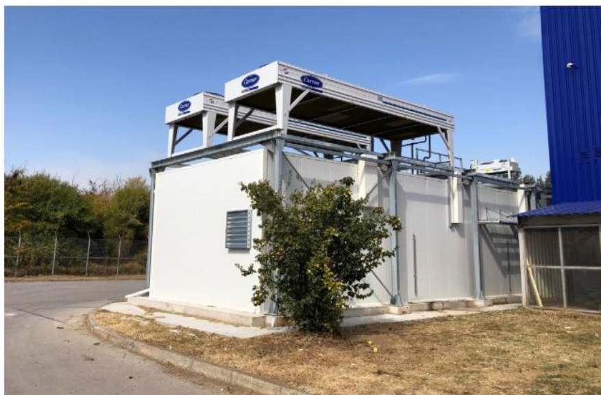
Outdoor CO 2 rack station
