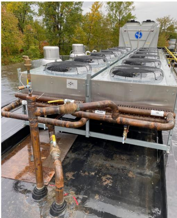
Ambient fluid cooler for heat of rejection from low-temperature R290 cases
