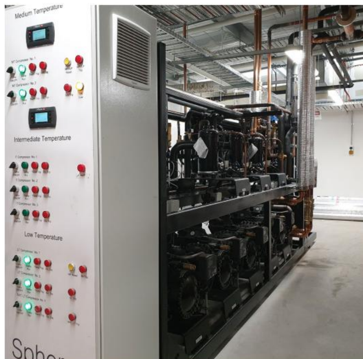
Transcritical CO 2 system at Michael's SUPA IGA store in Keysborough, Victoria.
