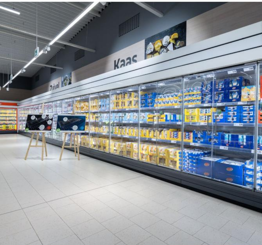
The refrigerated cabinets in the store are cooled by a Teko CO 2 rack.
