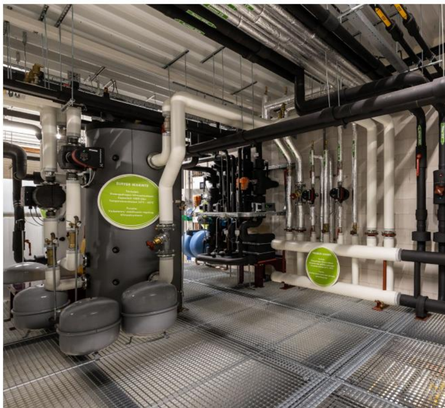
Hot and chilled water tanks for climate control of the store.
