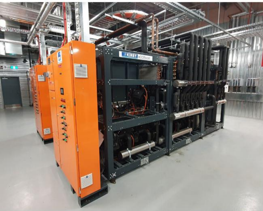
Two transcritical CO 2 racks from Kirby at the Woolworths Burwood store.
