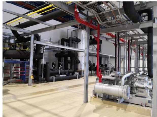
The ammonia machine room at L.A. Farm S.A.
