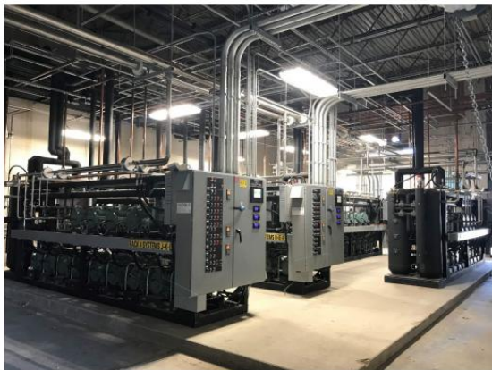
Inside the 4MW Yosemite refrigeration machine room.
