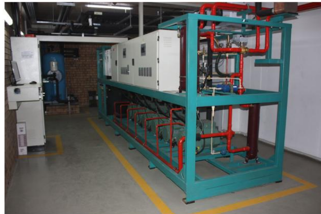
Inside the machine room of SPAR Wonderpark.
