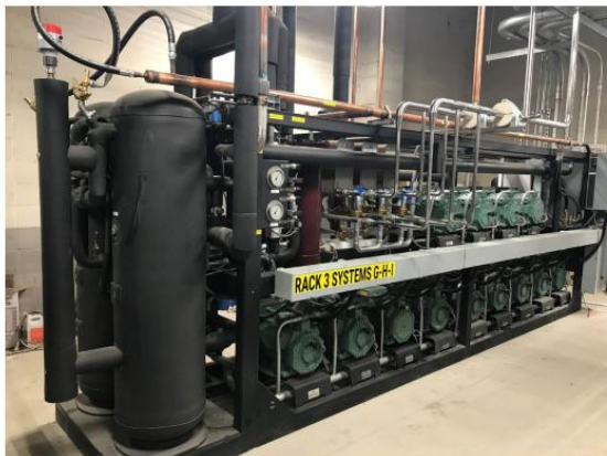
One of the CRS racks from Sphere Solutions up close.
