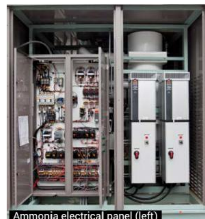
Ammonia electrical panel (left) and VFDs for ammonia compressors.
