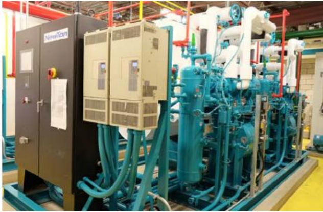
In Ontario, Canada, at the Toronto plant of Wholesome Harvest Baking, (2) NewTon R-6000 units (cooling capacity 54TR) are installed for their spiral freezer.
