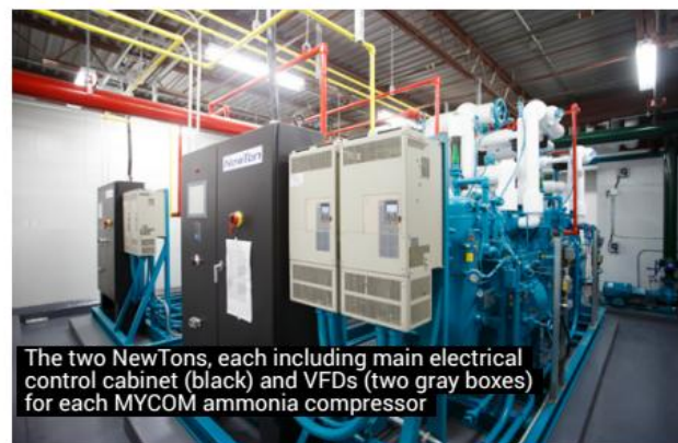
The NewTon, including emergency and controlled venting lines (red and yellow); glycol supply and return lines (dark green, at right)
