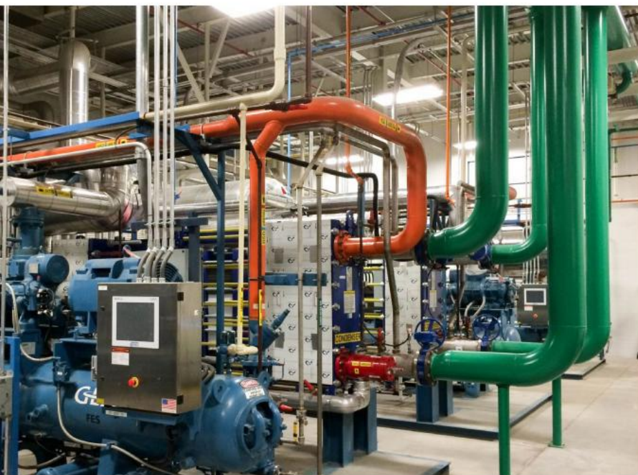
HVAC glycol low-charge ammonia chiller package in machine room at Pepperidge Farm plant, Richmond, Utah
