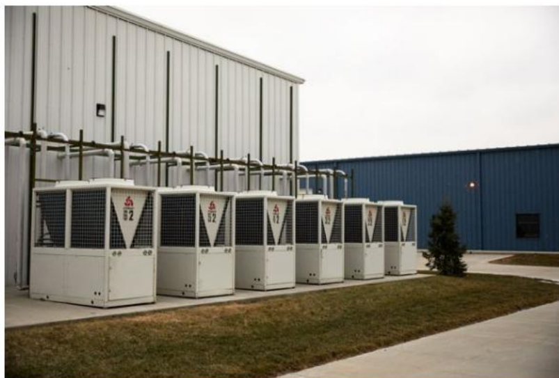
8 / Outside chillers for environmental chambers in adjoining building
