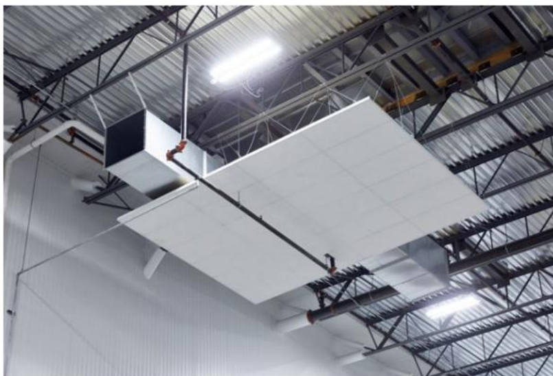
9 / Ducting from the NXTCOLD unit into the dock area
