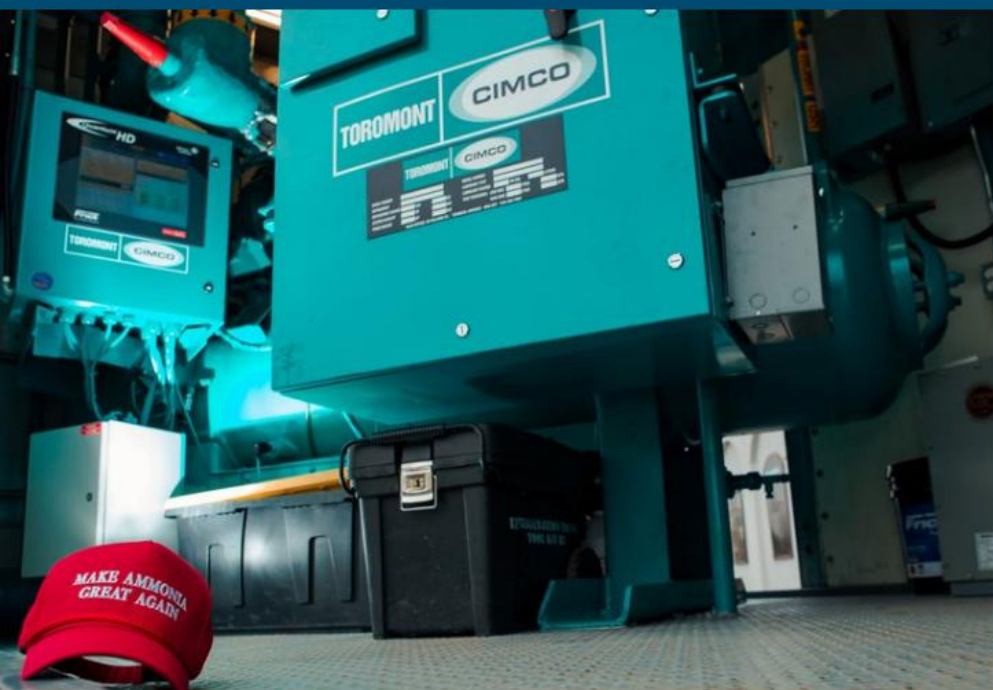
Ammonia equipment in CIMCO's mobile trailer used to make outdoor ice rinks for the NHL
