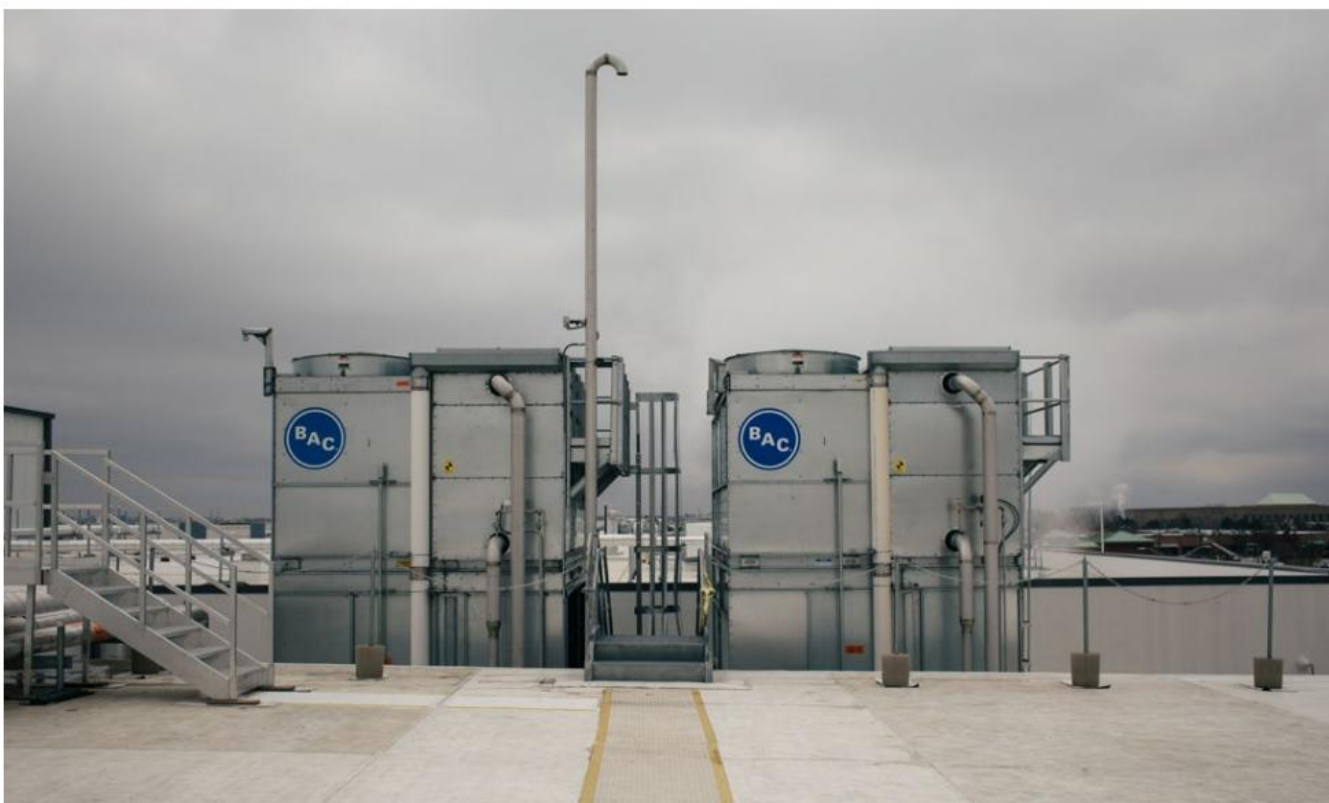
BAC evaporative condensers above the engine room
