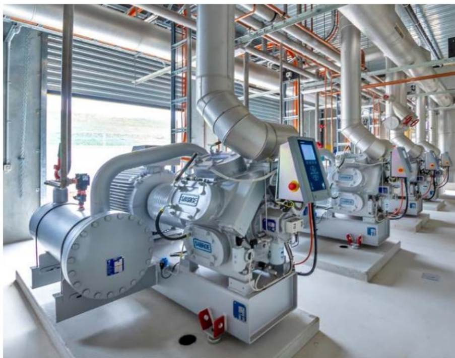
Scantec's central low-charge \text{NH}_3 (300 kg) plant room, in Brisbane, Australia
