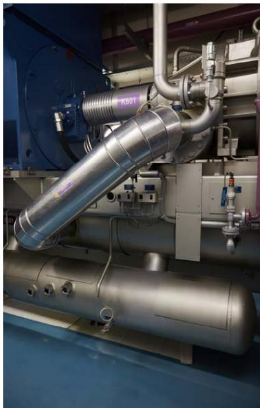
Parts of a Roche ammonia chiller installation in Basel, Switzerland.
