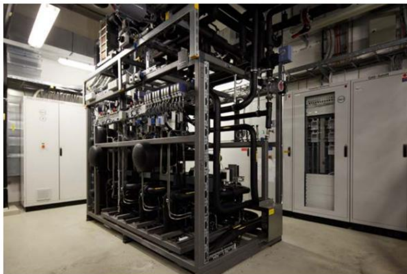
Roche's CO 2 transcritical double-stage system in Basel, Switzerland.
