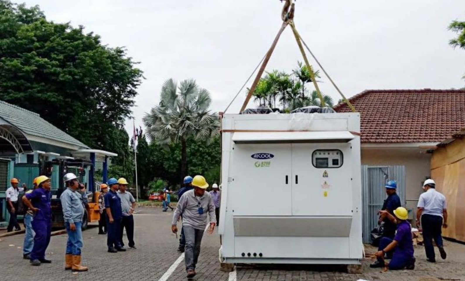
Placing of R290 chillers at the pharmaceutical company PHAPROS.
