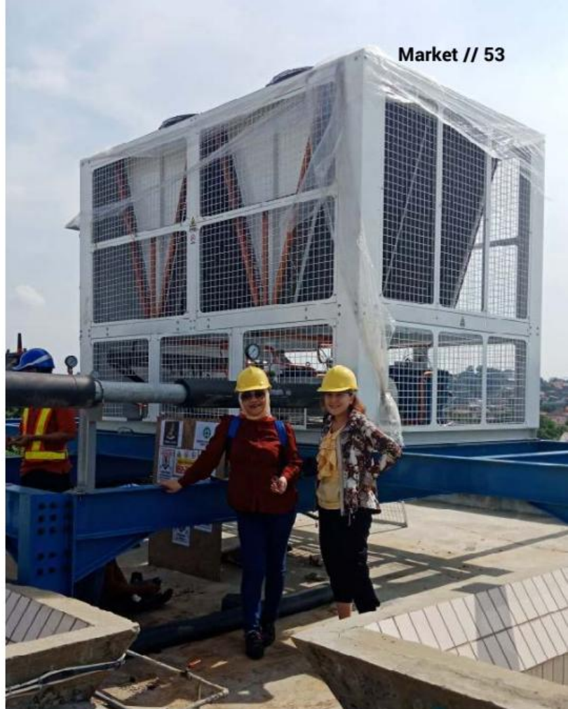
Herlin Herlianika and Indira Darmoyono (GIZ Green Chiller consultants) with the commissioned R290 chiller.
