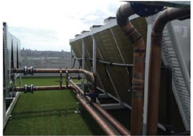
Hydraulic equipment and installation.
