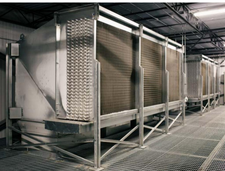
Penthouse DX evaporators.
