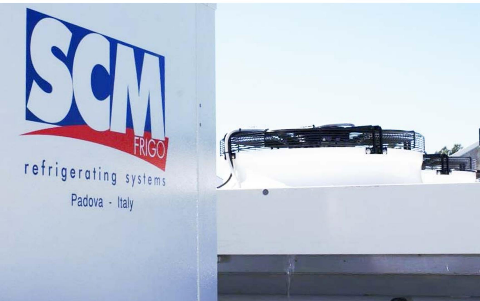
SCM Frigo transcritical CO 2 system with Luvata CO 2 gas coolers
