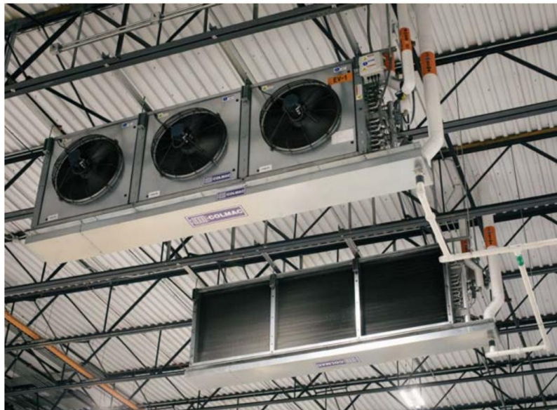
Hanging DX evaporators in dock area.
