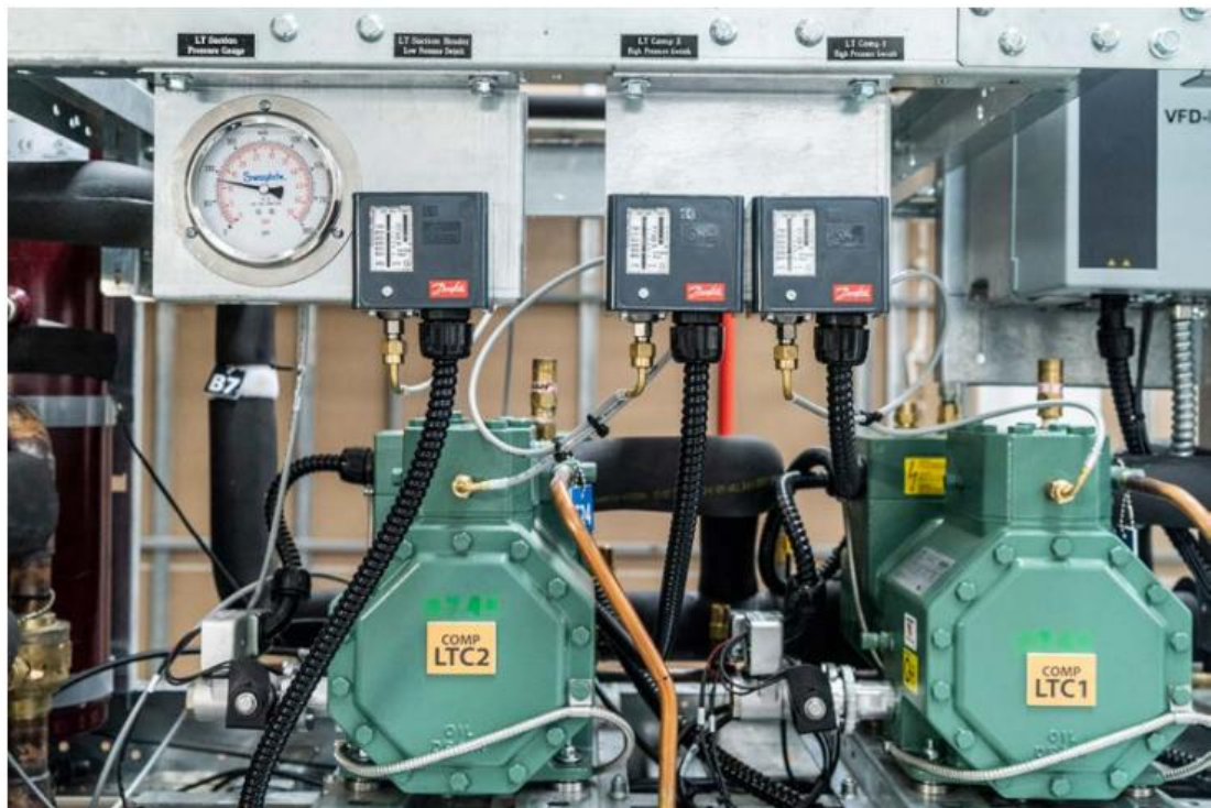
Kysor/Warren transcritical CO 2 rack, Culiacán store.
