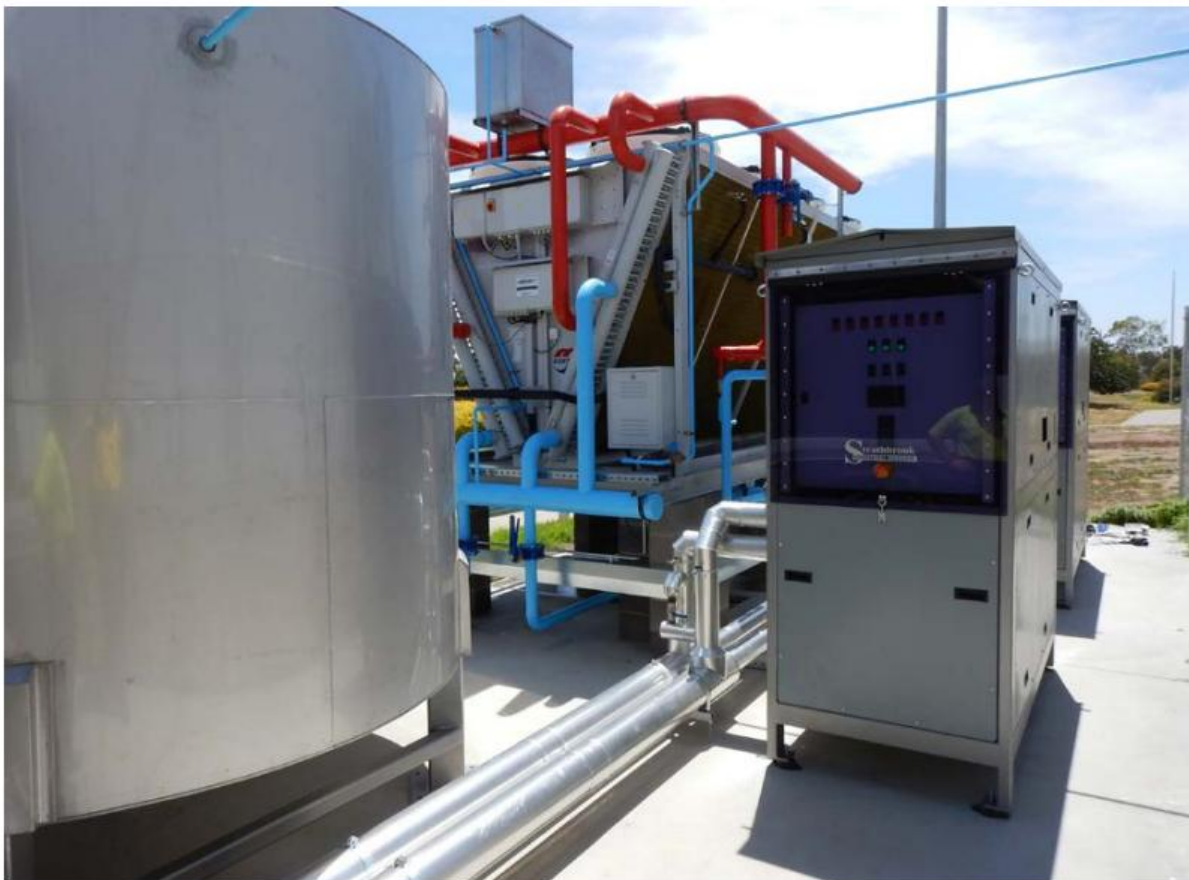
F. Meyer cold storage warehouse in Melbourne with CO 2 gas cooler and two ammonia chillers.
