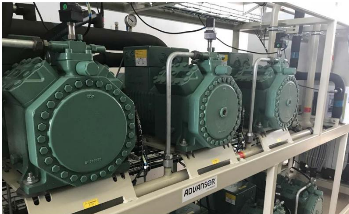
Advansor's first CO 2 transcritical rack in Australia in Keysborough, Melbourne, for a United Food Express cold storage warehouse.
