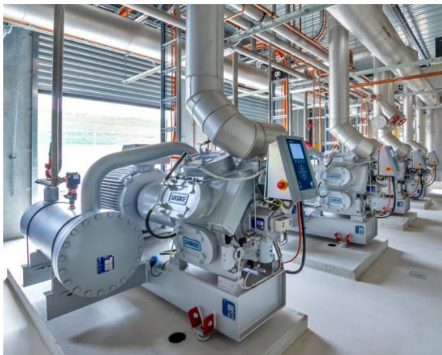
Scantec's central low-charge \text{NH}_3 (300 kg) plant room, in Brisbane.
