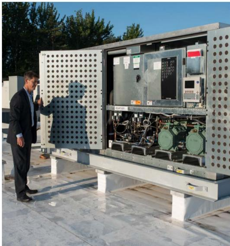
ALDI VP Aaron Sumida viewing inside of AdvansorFlex
