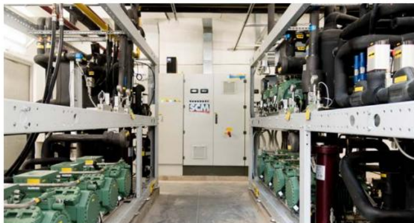
Transcritical CO 2 booster racks
