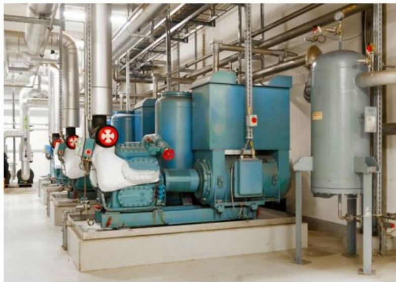
CO 2 engine room, Nescafé Factory (Orbe), Switzerland
