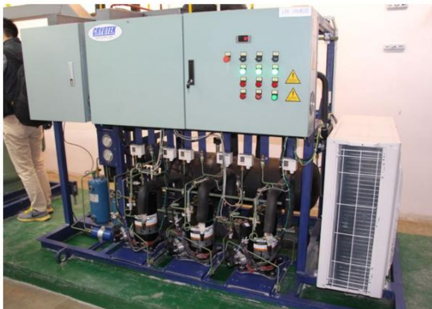
Low-temperature CO 2 rack
