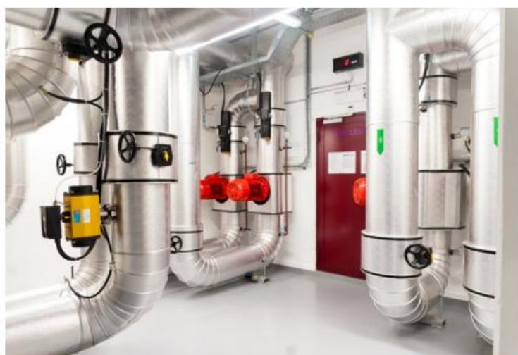
Ammonia engine room, data centre, Bussigny
