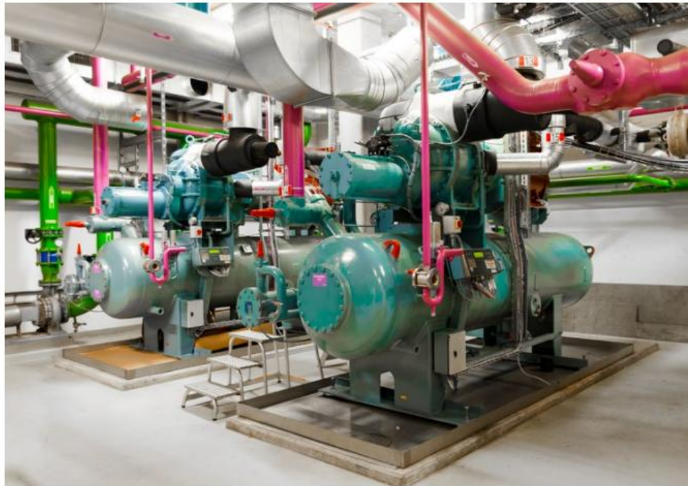
Ammonia engine room, Nescafé Factory (Orbe)
