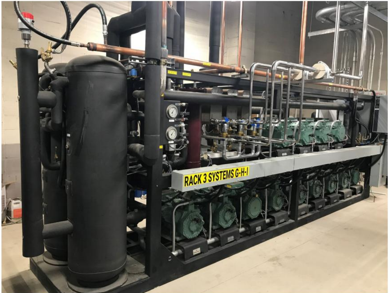
The refrigeration racks were all manufactured in South Africa.
