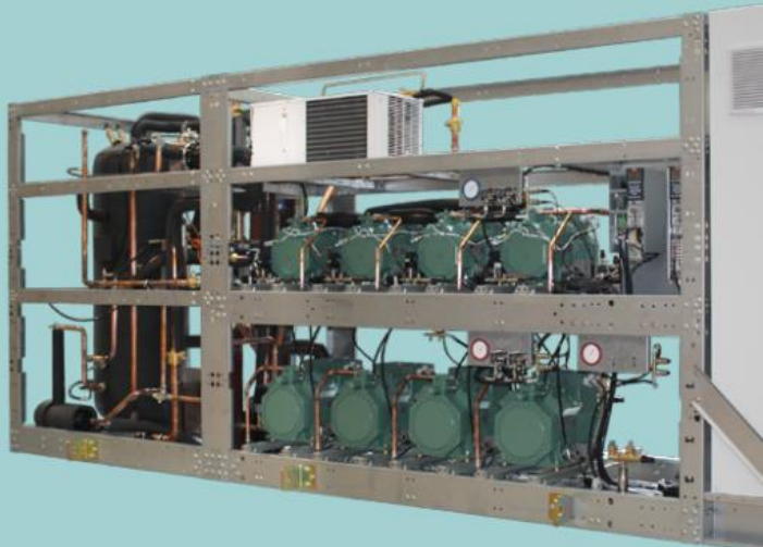
HK Refrigeration eCO 2 Boost transcritical system
