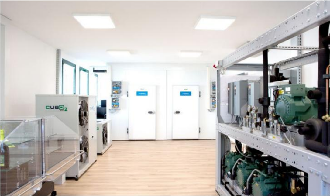
SCM Frigo's CUBO 2 Smart condensing unit (l) and a CO 2 transcritical rack (r) at the Beijer Ref Academy.
