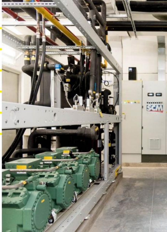
SCM Frigo CO 2 transcritical rack in METRO China's Beijing Lishuiqiao store.
