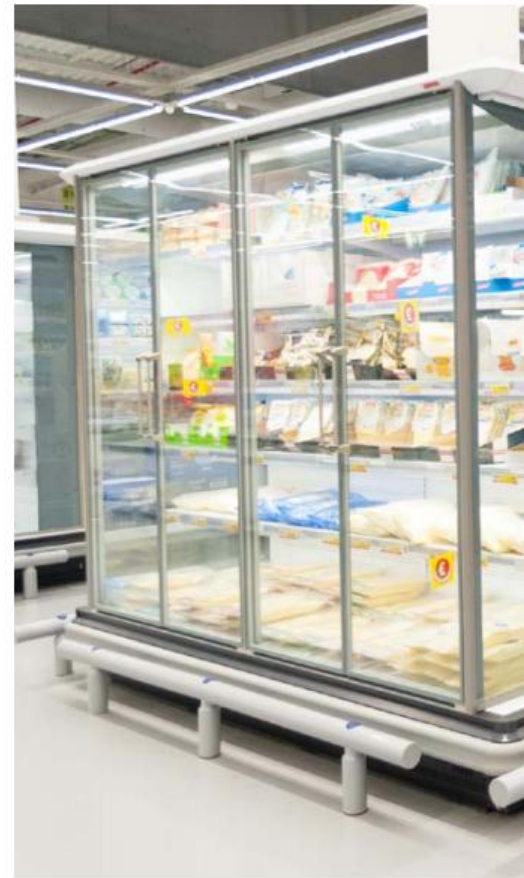
1 & 2 / In the Sines store, the Advansor CO 2 transcritical rack serves large freestanding and wall-mounted cabinets and a cold storage space.
