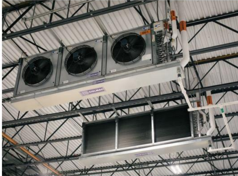
Hanging DX evaporators in dock area.
