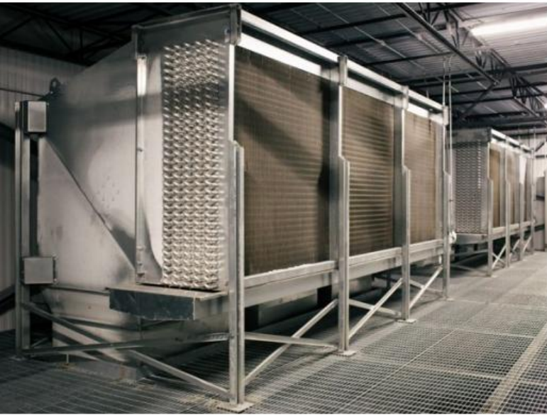
Penthouse DX evaporators
