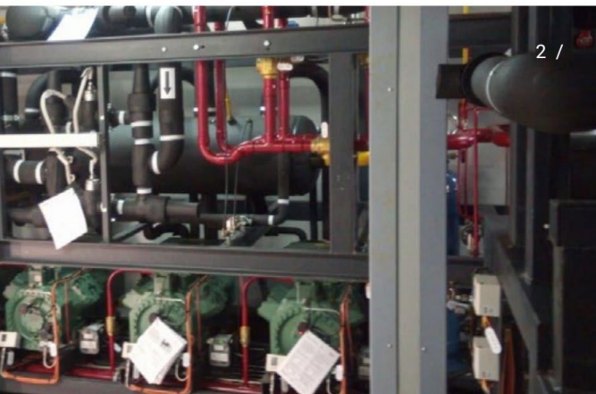
1 / Güntner gas cooler on the roof of Aparinki store. 2 / CO 2 transcritical rack, Aparinki.
