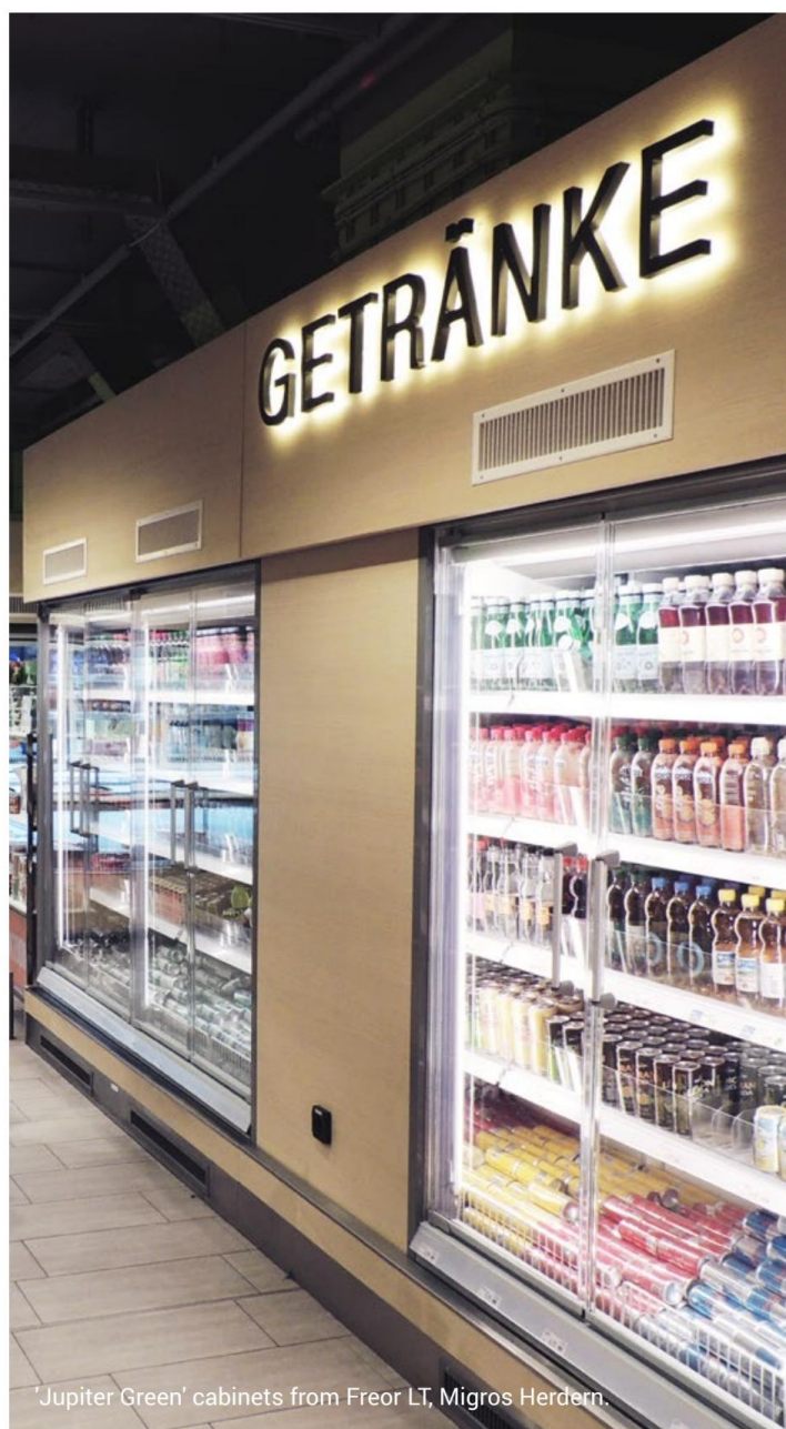
Migros Herdern, where the retailer's pilot propane water-loop system was installed in May 2016.
