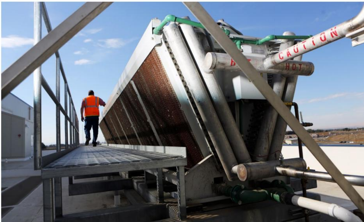
Liquid and suction CO 2 pipes for freezer evaporators
