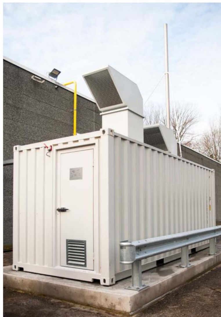
Combined heat and power plant, Pummerend store
