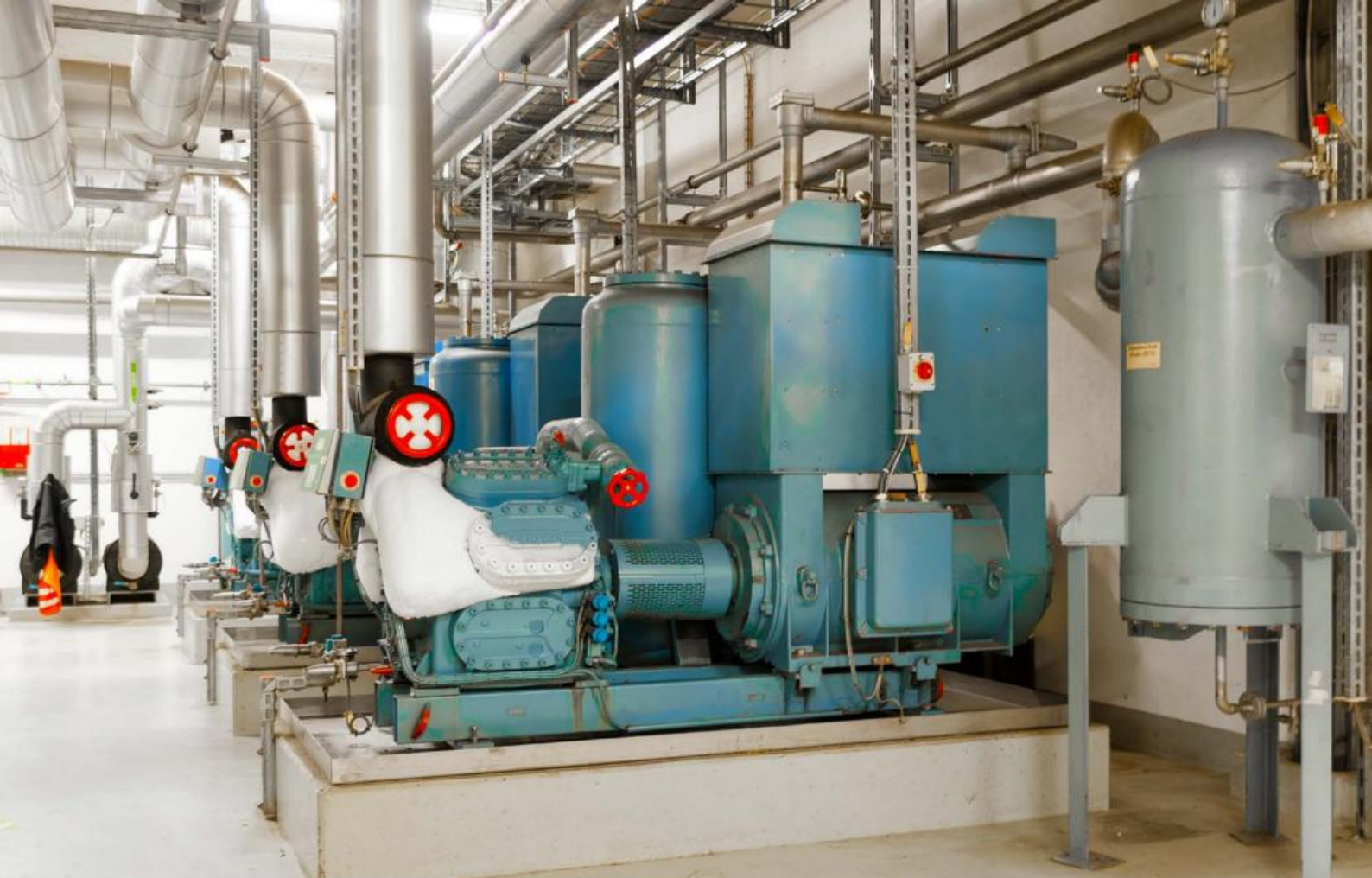
CO 2 engine room with HPC 108S reciprocating compressors from Sabroe (JCI) operating at -54°C. Nescafé Factory (Orbe).
