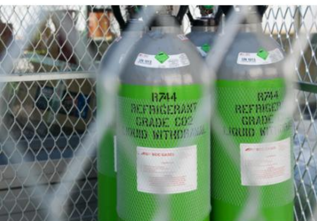
Above and below: The system uses natural refrigerants ammonia and CO 2
