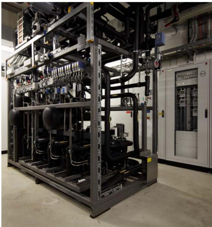
Installation 1: CO 2 transcritical double-stage system.
