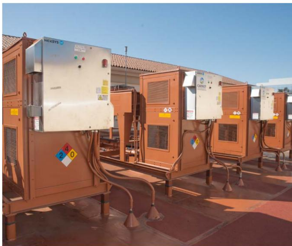
Medium-temperature propane chillers on the roof of Whole Foods' Santa Clara, Calif., store
