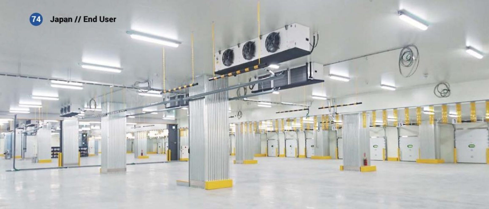
CO 2 unit coolers inside Kokubu's Kawaguchi distribution center
