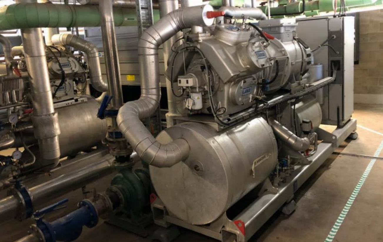
Two ammonia-based chillers providing air conditioning for the Logan City council administration center in Queensland, Australia
