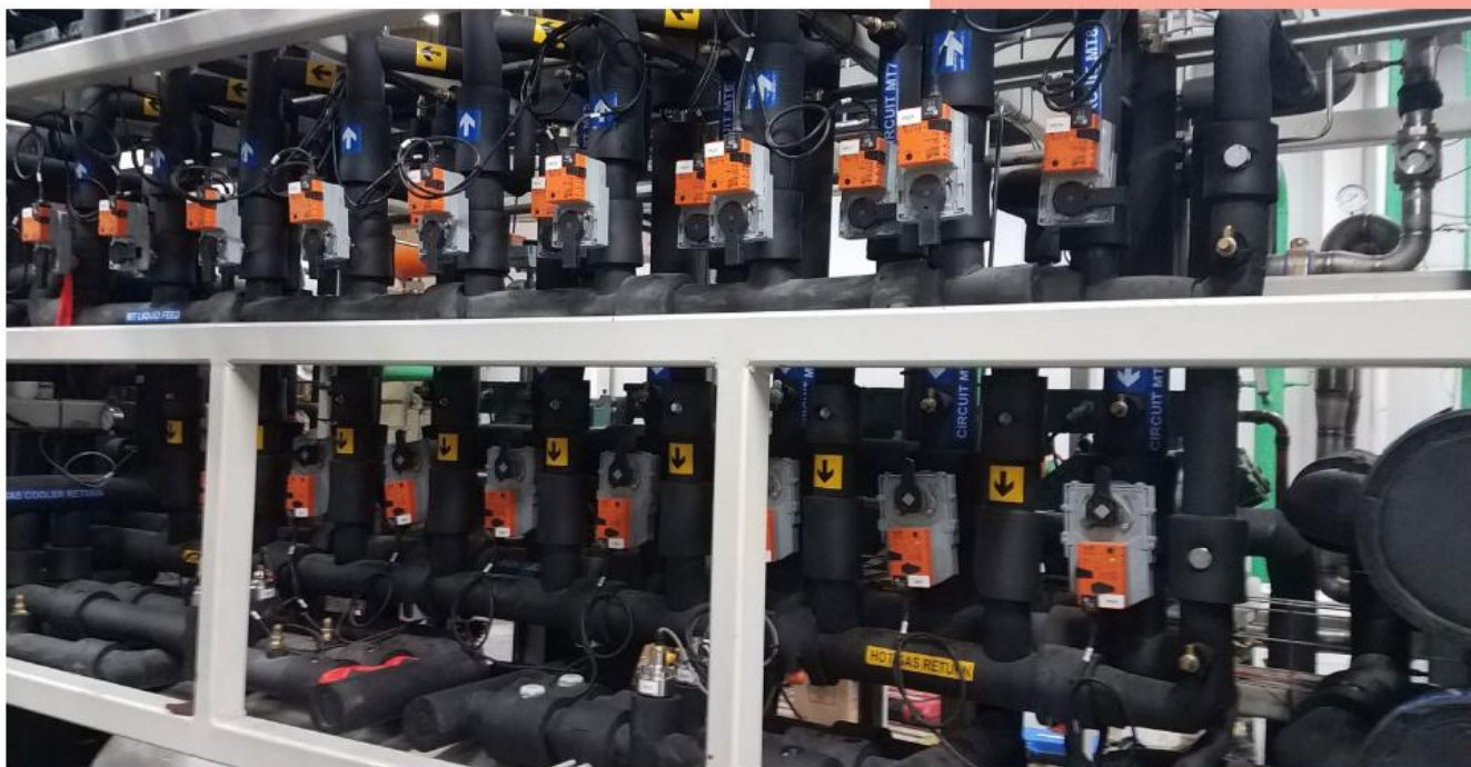
Medium-temperature CO 2 rack at Hannaford warehouse.
