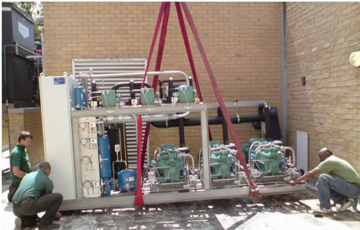
The PnP Strand CO 2 refrigeration rack arriving on-site.
