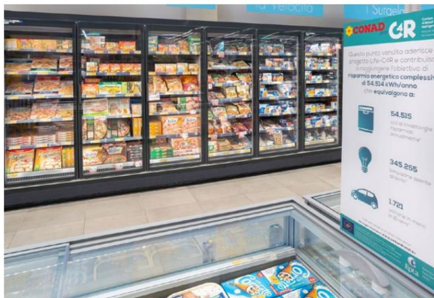
Epta's first Italian pilot system for Life-C4R project
