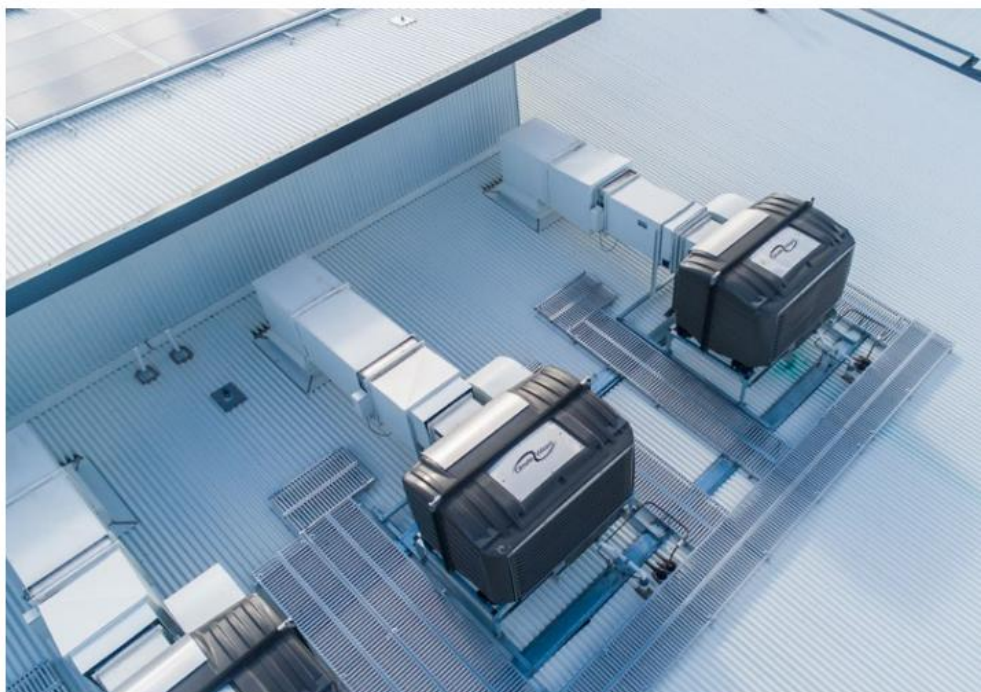
Climate Wizard machines installed on a roof.
