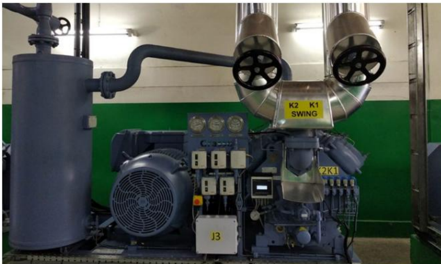
GEA Africa supplied the compressor sets and other refrigeration equipment.
