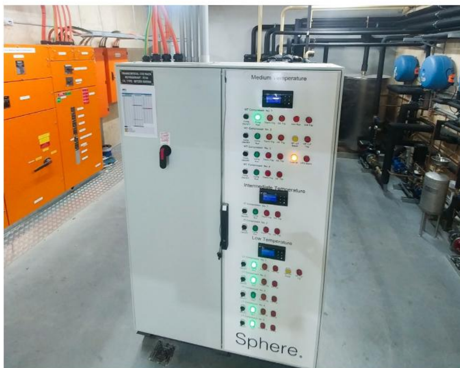
Controls for transcritical CO 2 rack
