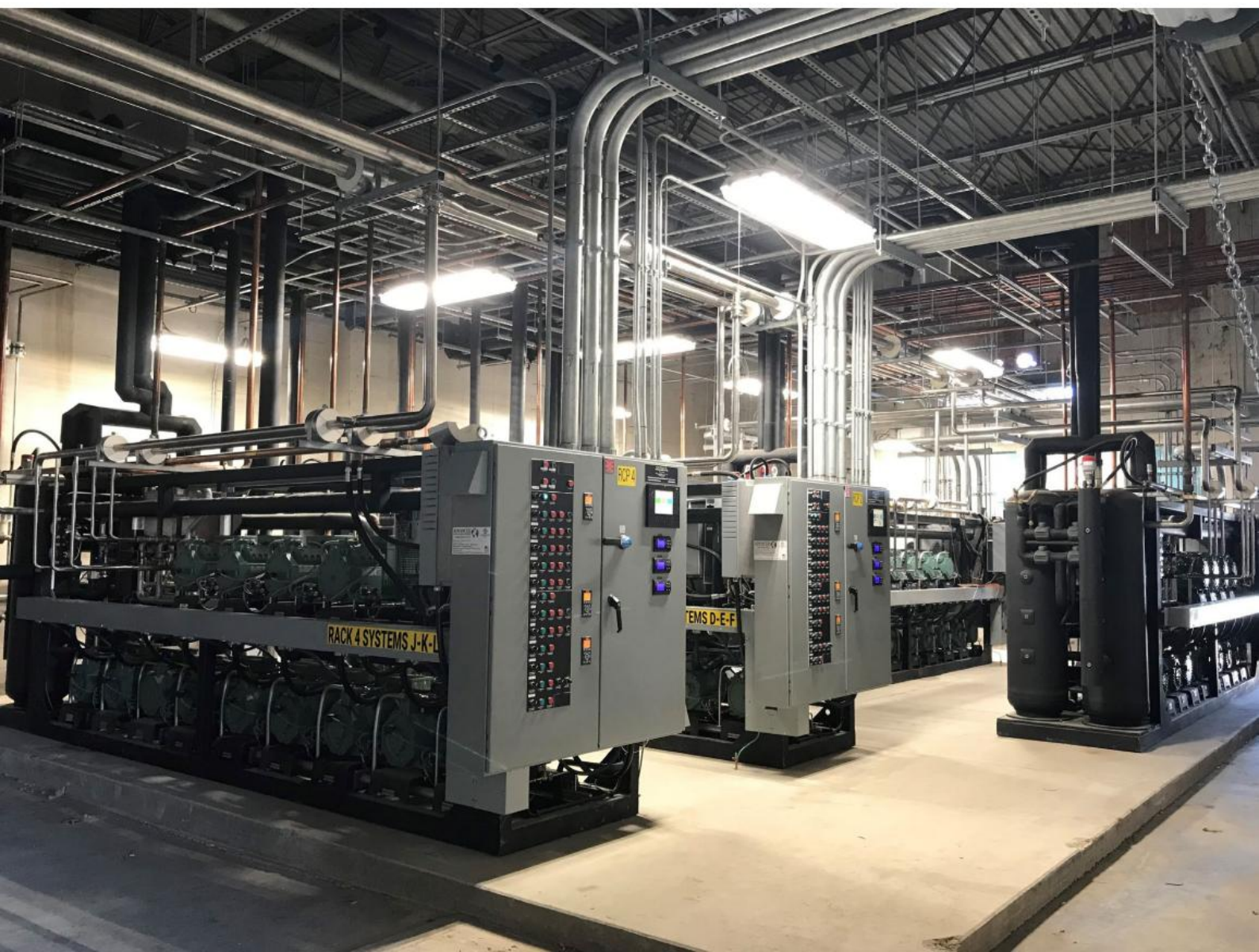
Five CO 2 racks are used at Yosemite Foods.
