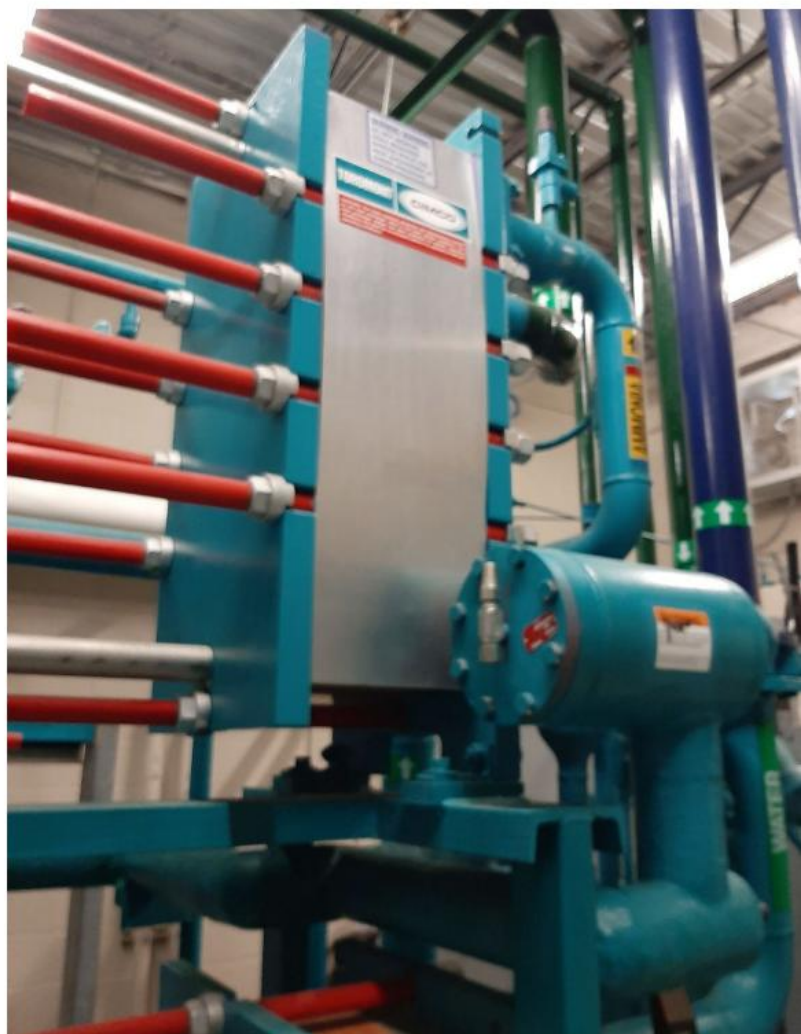
Alfa Laval heat exchanger for transferring heat from ammonia to glycol
