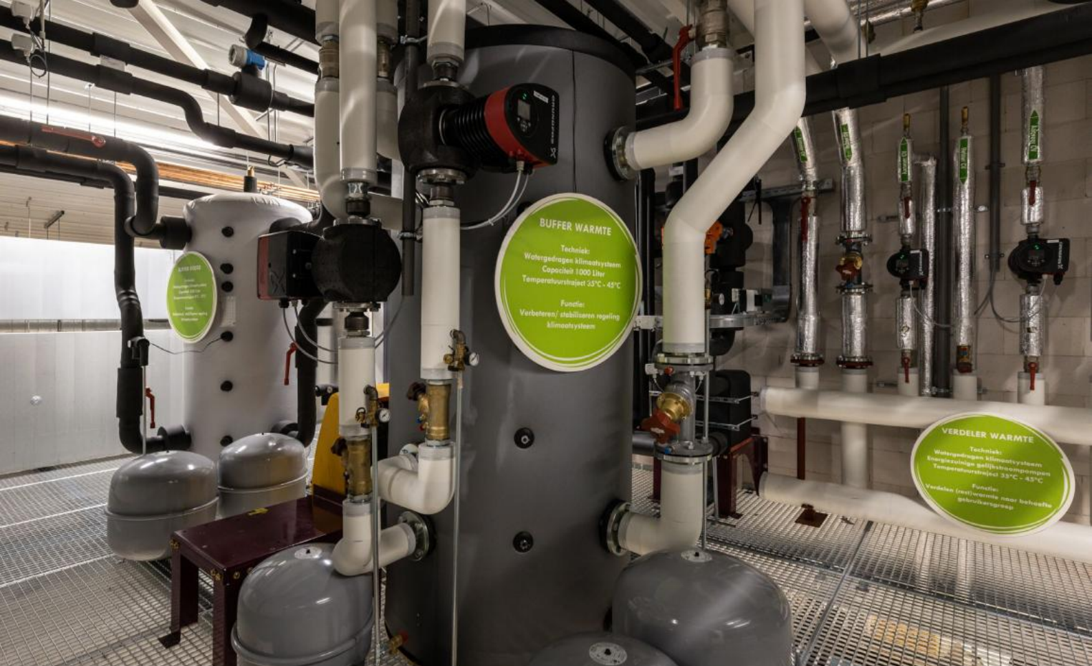
Hot and chilled water tanks for climate control of the store.
