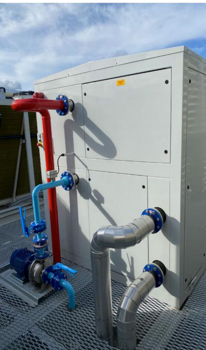
SCM Frigo's NH 3 Aqua Ultra Chillers and condenser water pump.
