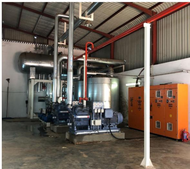
The upgraded ammonia system at Afrupro.
