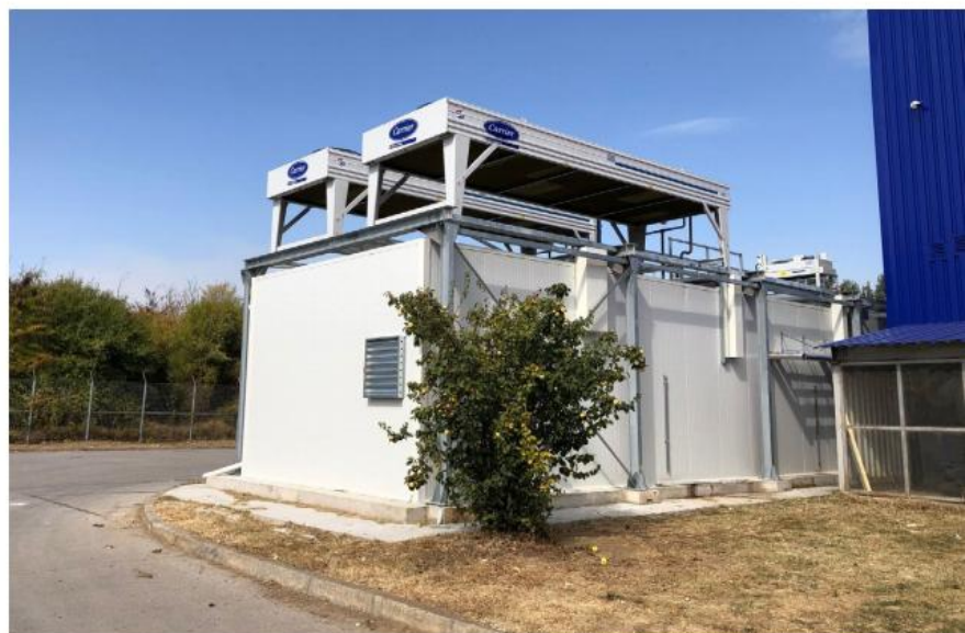
Outdoor CO 2 rack station
