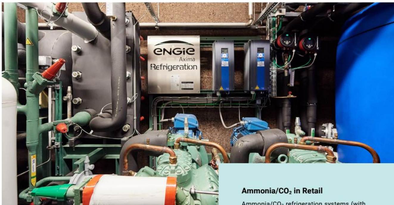
Part of the ammonia refrigeration rack used by the ammonia/CO 2 /glycol system in a Delhaize store in Belgium
