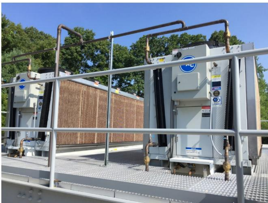
Two adiabatic gas coolers for transcritical CO 2 system at Weis store
