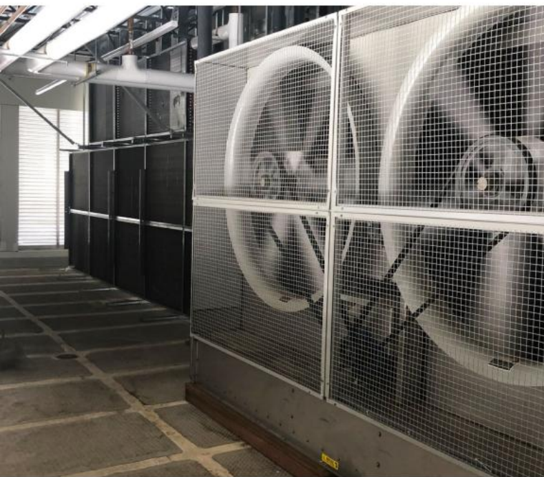
Water tower/air fluid cooler
