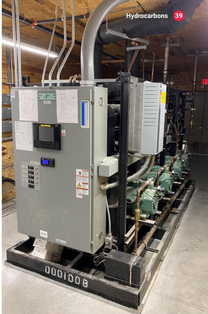
Transcritical CO 2 /glycol chiller for medium-temperature loads
