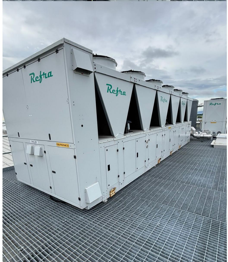
Refra's heat pump (up) and chiller at Keelings' flower processing facility in Dublin. Photo credit: Anglo Irish Refrigeration
