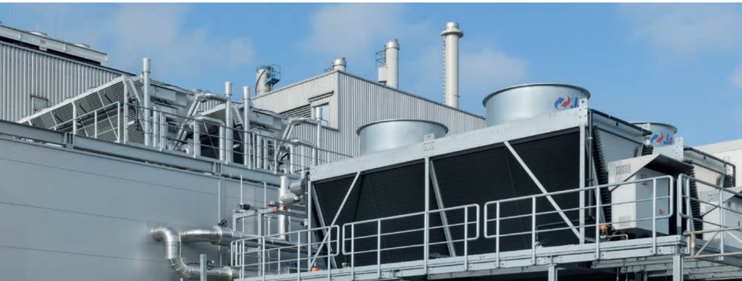
Jaeggi's hybrid dry cooler. Photo credit: Jaeggi.
