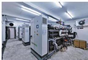
Heat pump in the abattoir of Zurich
