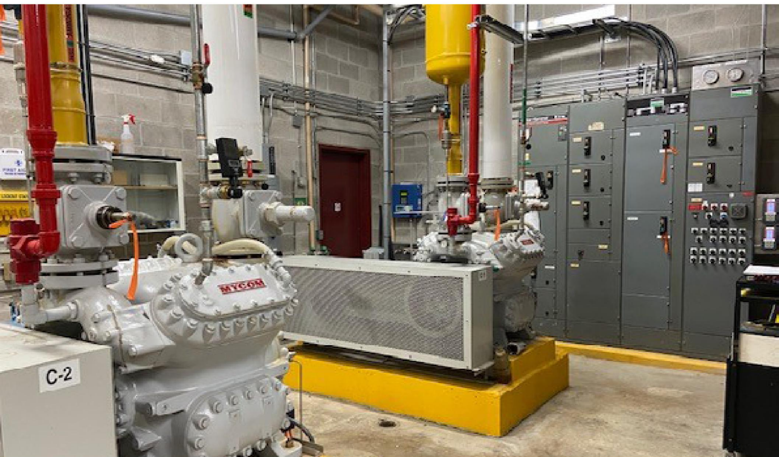
Compressor room, Pickering Ice Arena
