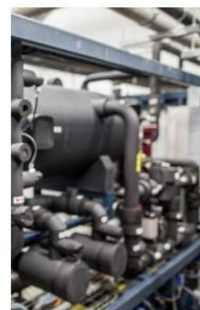
Equipment shot of a CO 2 transcritical rack
