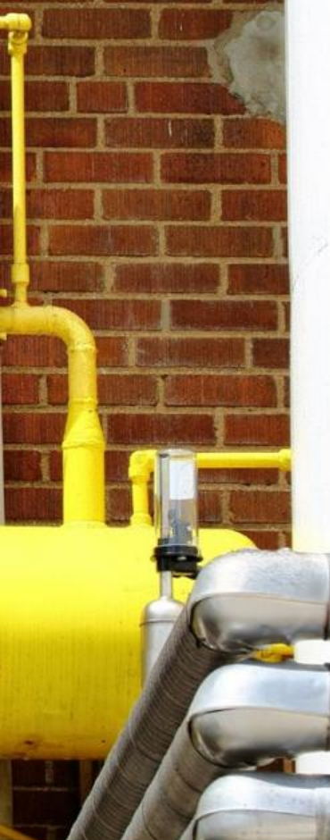
Above: Ammonia refrigeration piping and tanks
