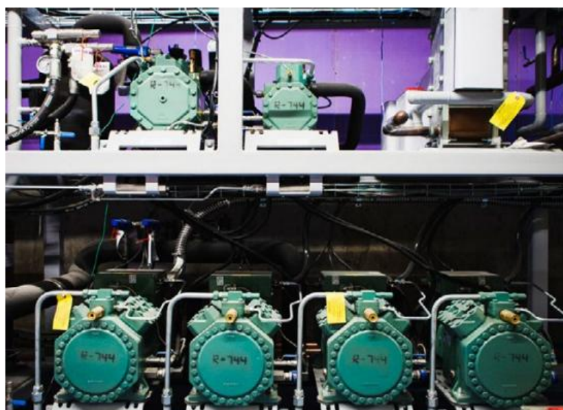
Compressors on a CO 2 transcritical rack
