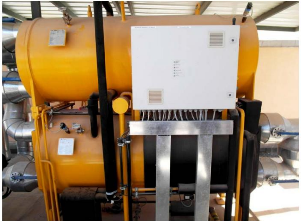
Absorption chiller 'Bumblebee'
